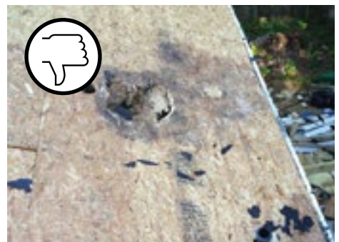
Dry rot or other damage
